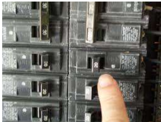
Reset Circuit Breakers
