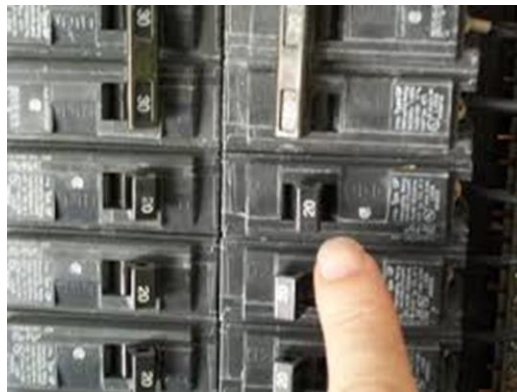
Reset Circuit Breakers
