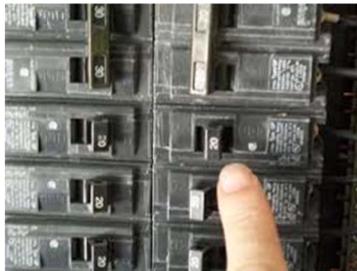
Reset Circuit Breakers
